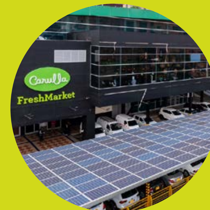
Painéis solares no Carulla Fresh Market
